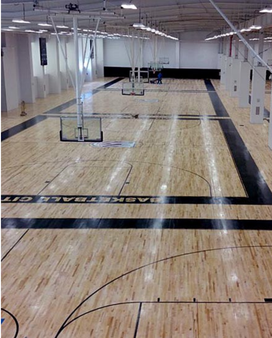
Seven air-conditioned basketball courts installed by AFR at Basketball City in NYC
